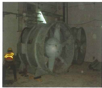
4 Hrs FRP 250°C Tunnel Fans
