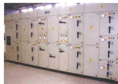
Motor Control Panel
