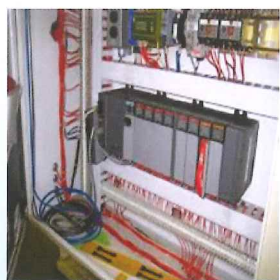
PLCs Cubic For Control
